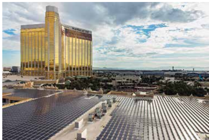
This solar array, one of the largest in the world, takes up nearly 20 acres of roof space atop the Mandalay Bay Convention Center.
